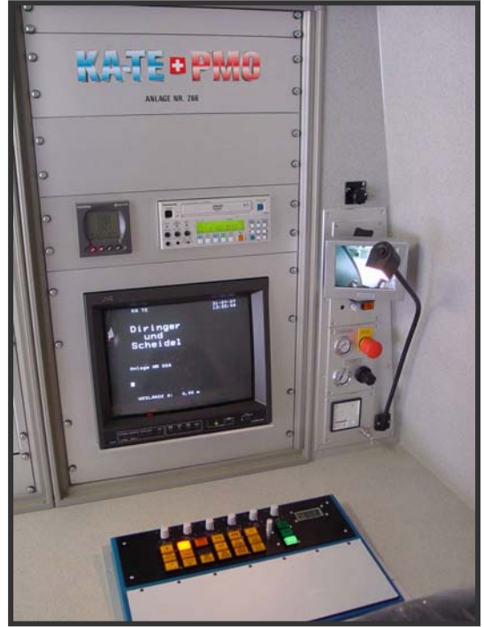
Cockpit: Controls, Monitor, On-Screen-Data, DVD Recorder, Monitor for Backroom Camera.
